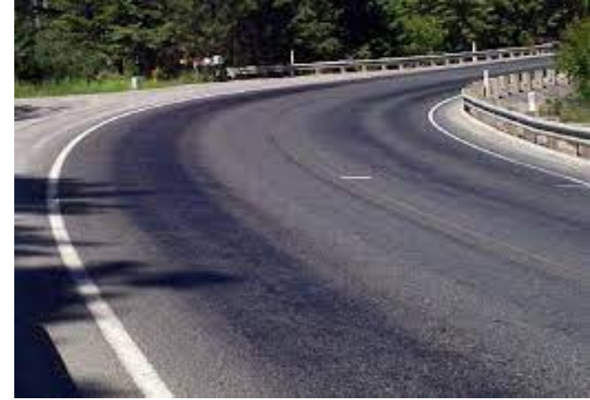
Flushing from maintained high temperatures and excess traffic volumes causing unsafe conditions.
