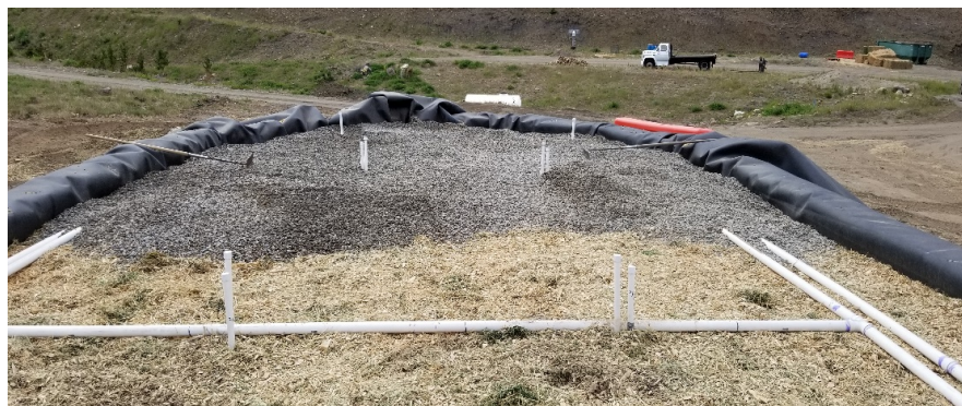
Biochemical Reactor Media Beneath Gravel Layer
