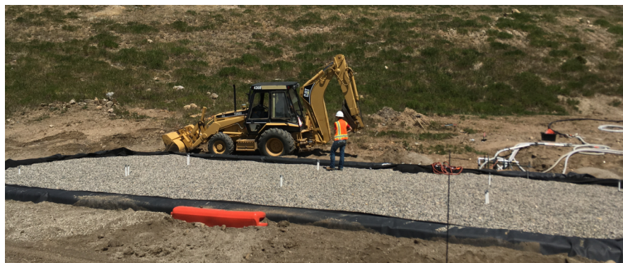
Biochemical Reactor Cell
