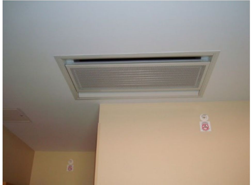
Chilled beam air distribution supplements radiant slab
