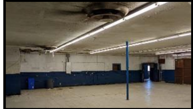
#3 Inadequate & Damaged Component Shop
